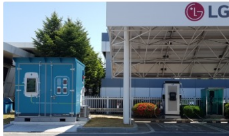
Korea Ochang Energy Plant
