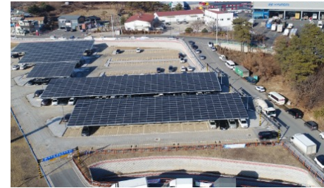
Cheongju Hope Green Power Plant
